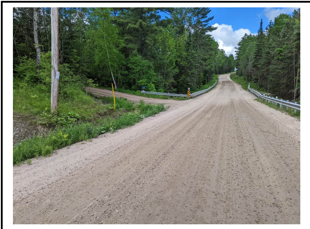
Photo 8 Tire rutting noted on east approach wearing surface
