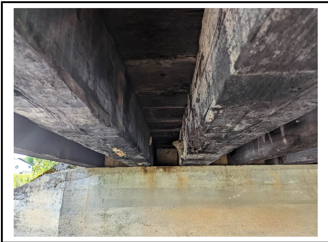
Photo 10 Weathering on timber girders
