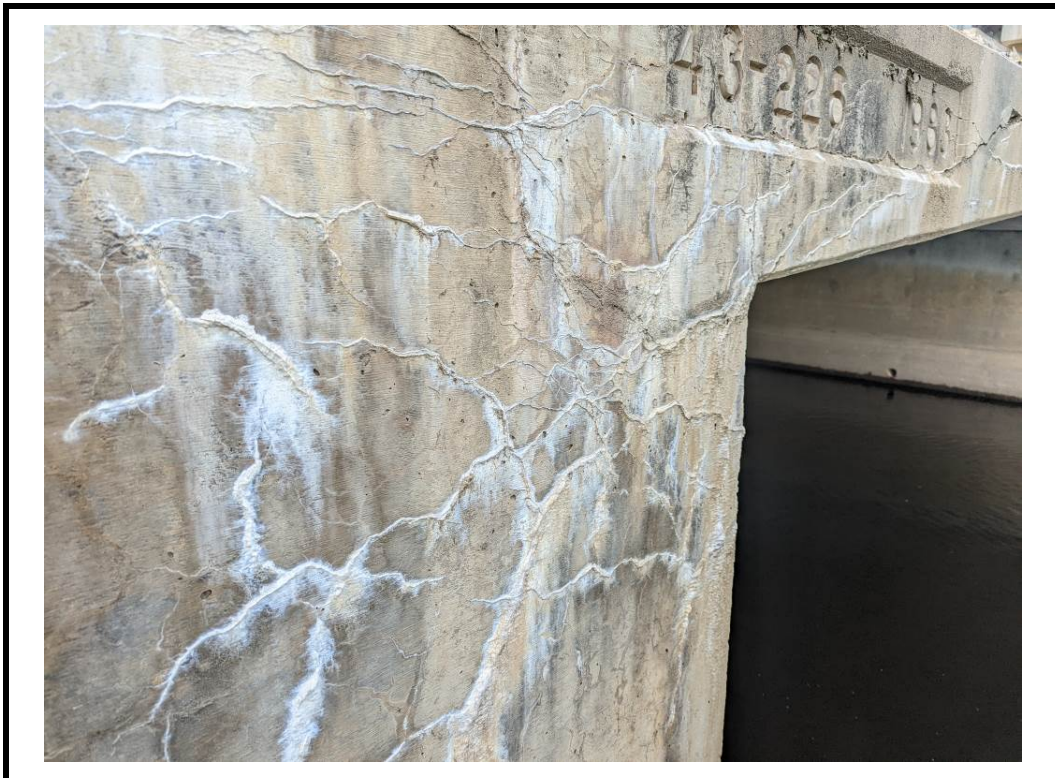
Photo 8 Narrow crack with efflorescence and rust stains on southwest wingwall
