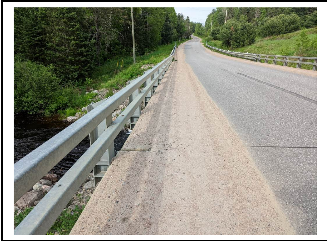
Photo 11 Sand accumulation noted on both side of deck wearing surface
