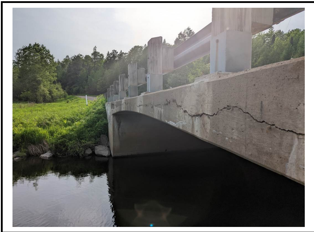
Photo 10 Wide horizontal cracks with concrete delamination noted on soffit exterior
