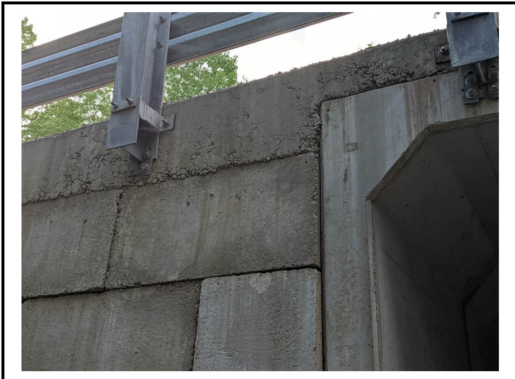
Photo 10 Light honeycombing noted on exterior deck soffit at northeast corner
