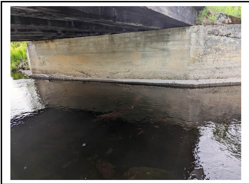
Photo 12 Moderate scaling on base of north abutment wall
