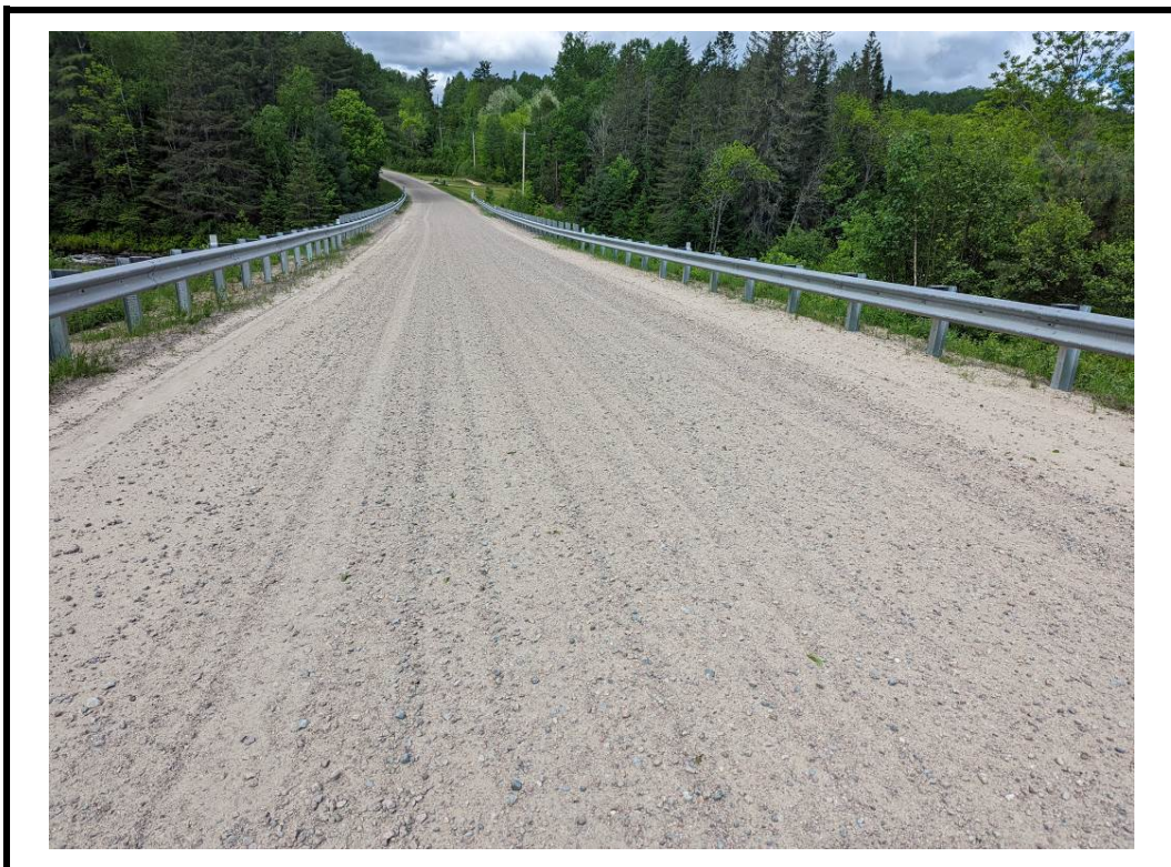
Photo 8 Light tire rutting and loose gravel noted throughout approach wearing surface
