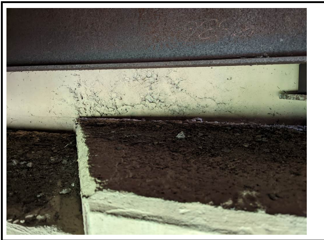
Photo 16 Light honeycombing noted on west ballast wall
