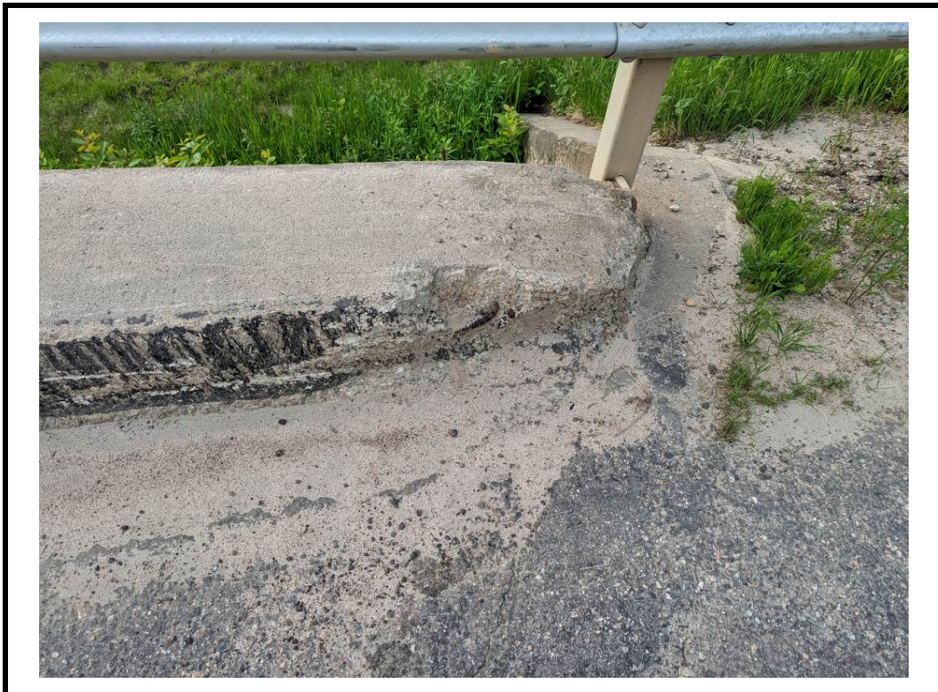
Photo 8 Small Spall with exposed corroded reinforcement noted on curb at northwest corner
