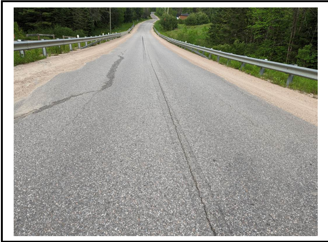
Photo 7 Wide transverse and longitudinal cracks on west approach wearing surface
