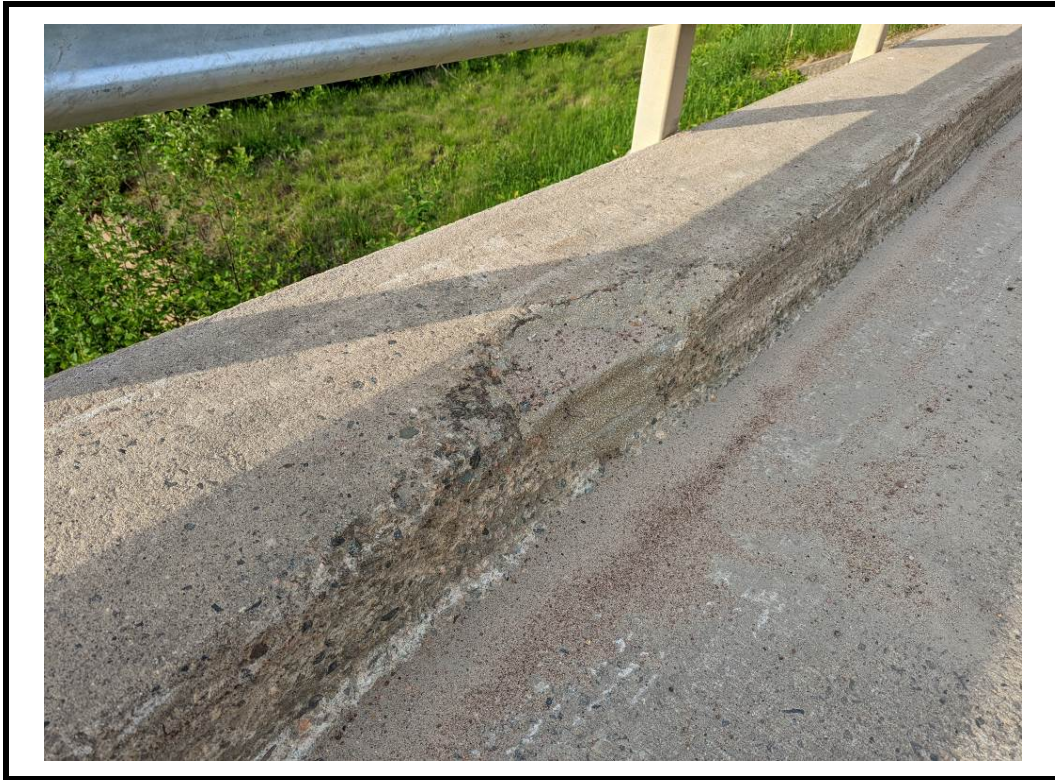
Photo 9 Scaling and abrasions noted on south curb
