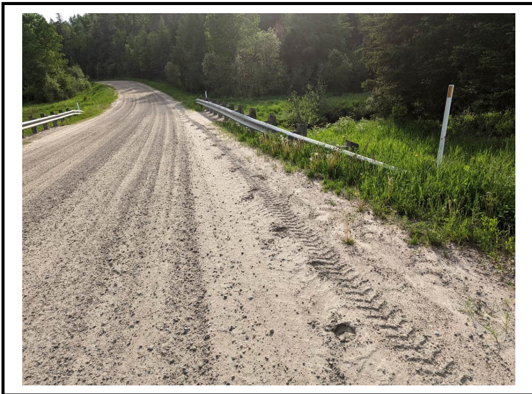
Photo 12 Moderate vegetation grown in front of approach guiderail
