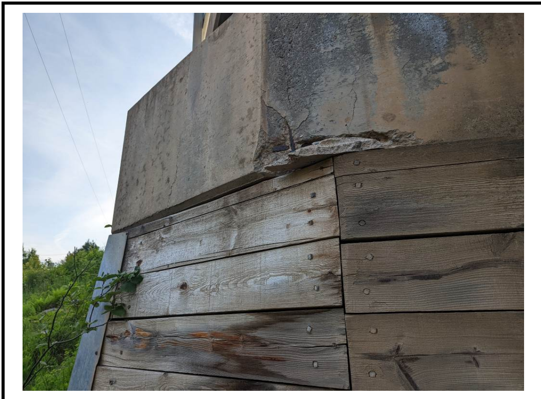
Photo 10 Spall with exposed corroded reinforcement noted on west pier cap
