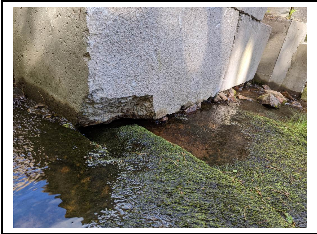
Photo 11 Some undermining and water flowing at southeast wall
