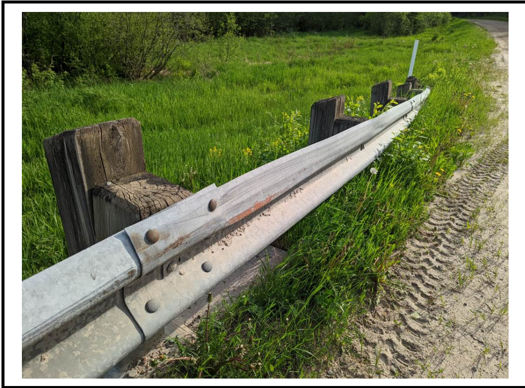
Photo 7 Substandard end treatment with damage northwest approach barrier
