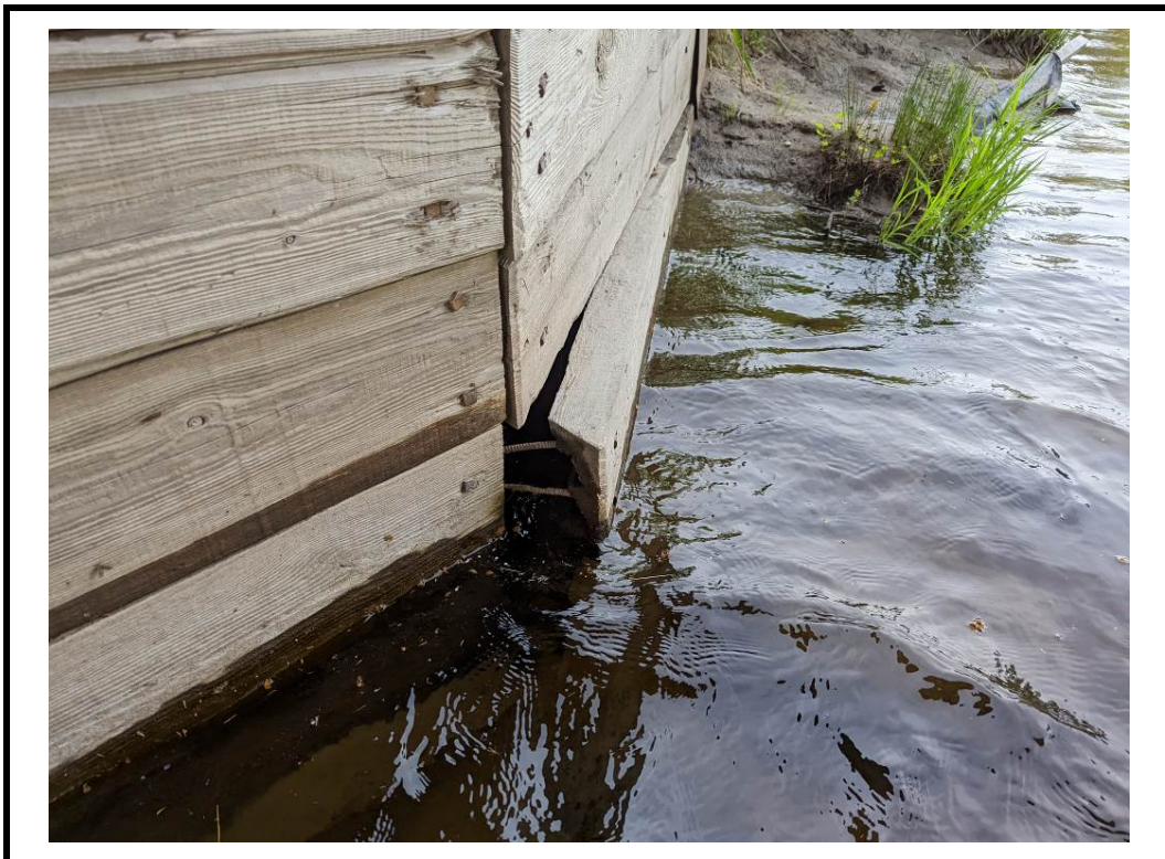
Photo 18 Some separation and weathering of timber crib noted throughout pier shaft
