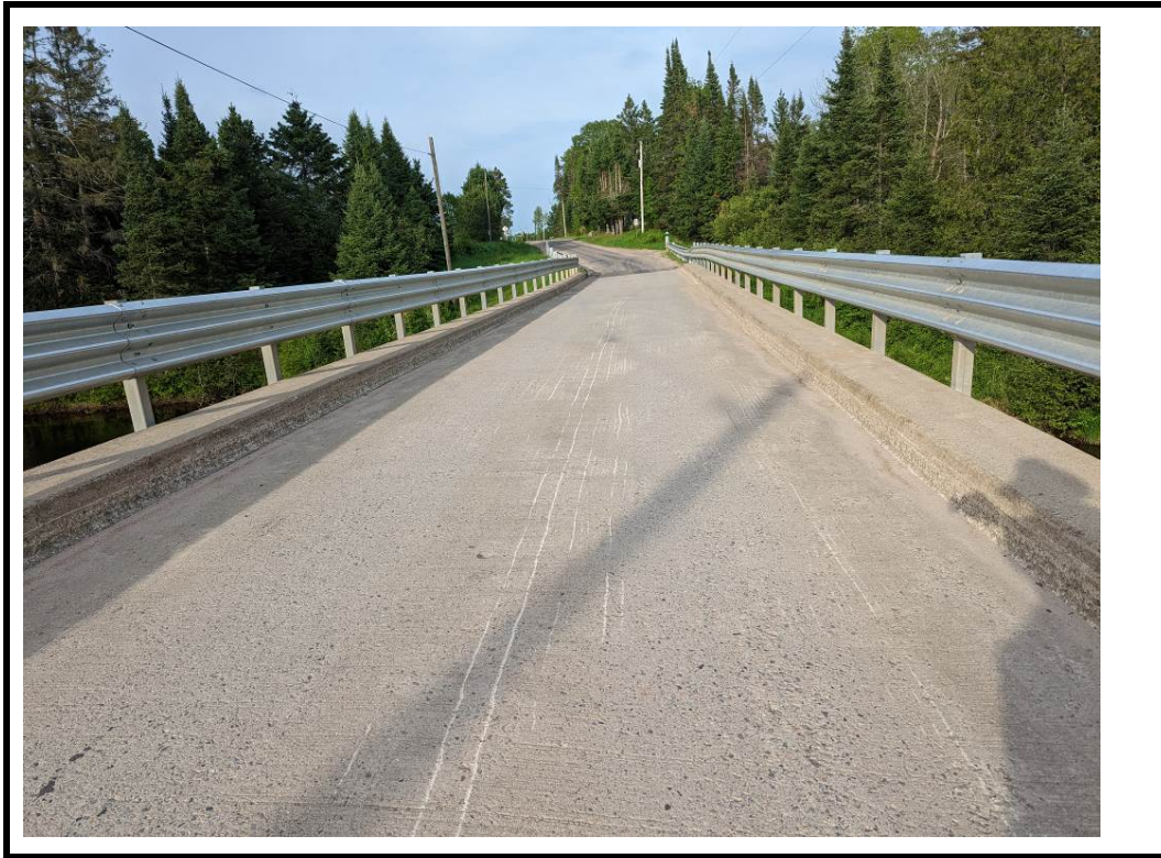
Photo 17 Light scaling and minor abrasion noted throughout exposed deck top
