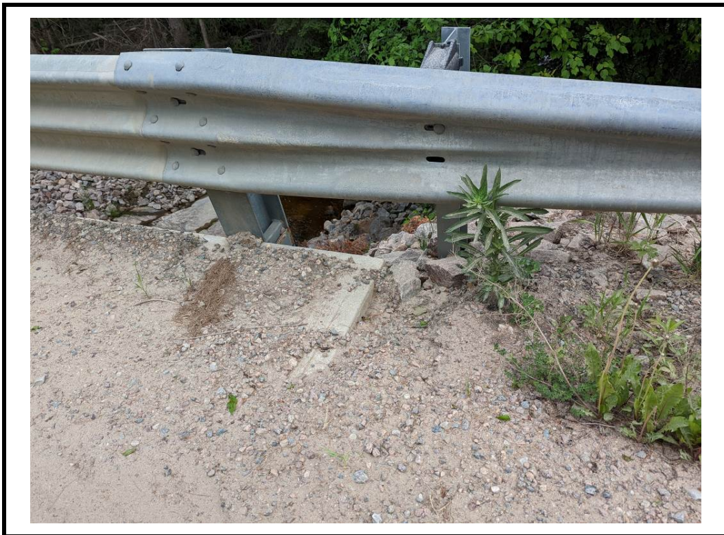
Photo 14 Some loose gravel noted at the edge of deck
