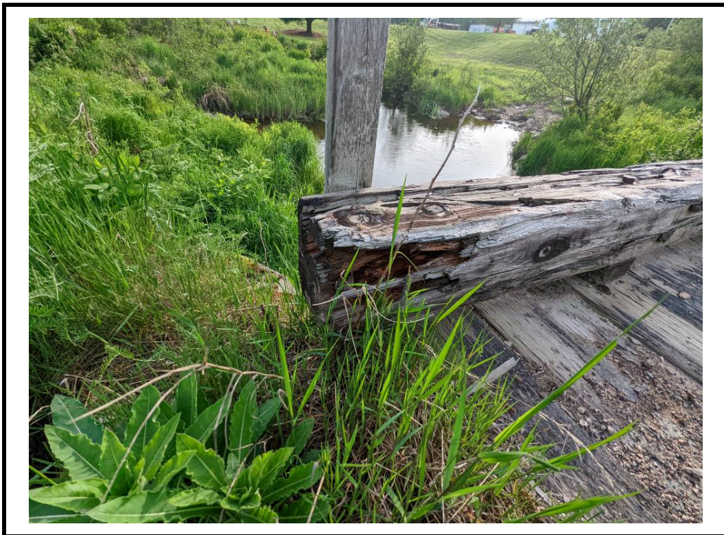
Photo 8 Splits, checks and rot on northwest timber curb
