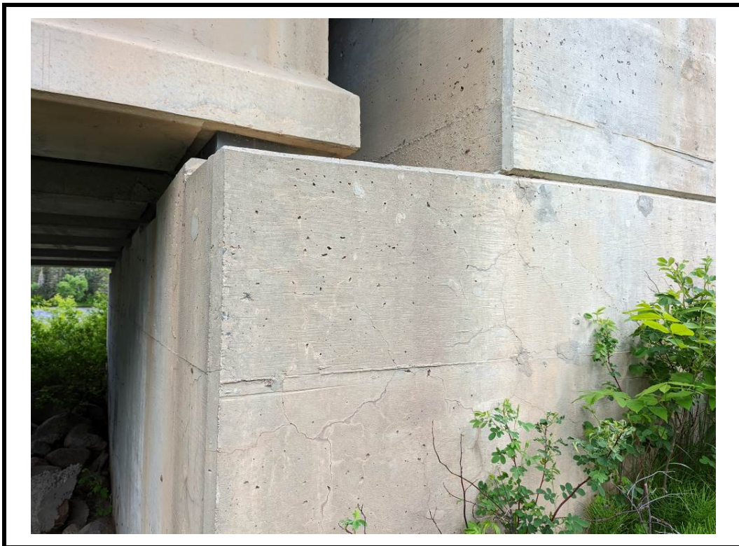
Photo 12 Cracks and stains noted on southeast wingwall
