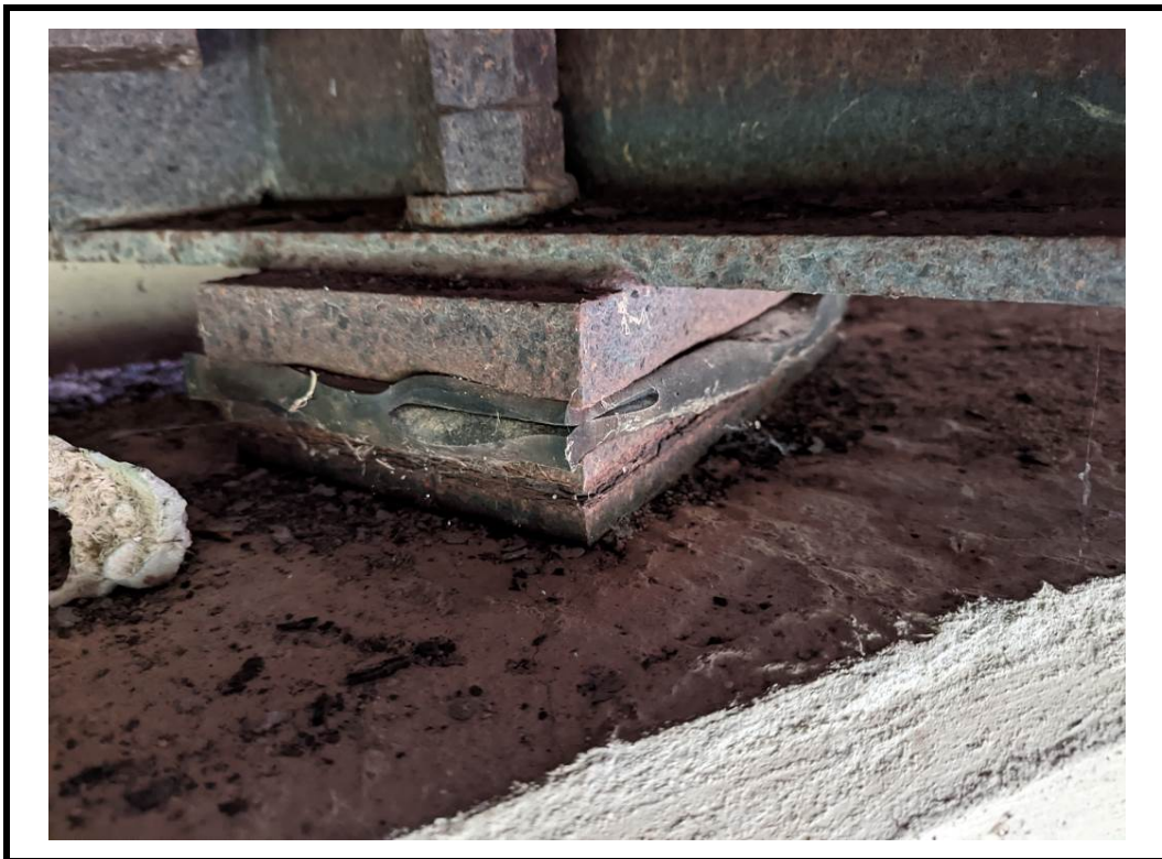
Photo 12 Bulging abutment bearing and corrosion on bearing plate at southwest corner
