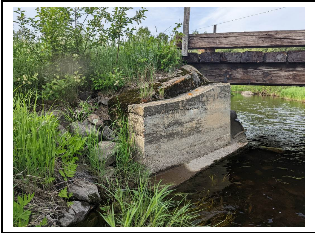
Photo 11 Moderate scaling noted on NW wingwall
