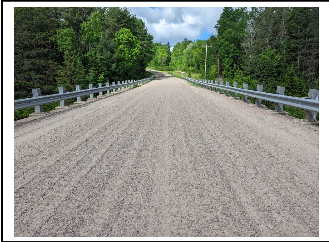
Photo 9 Typical deck wearing surface with loose gravel noted throughout
